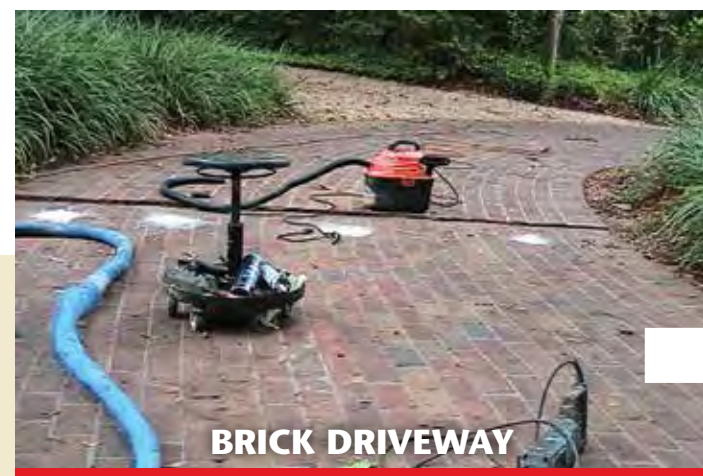
BRICK DRIVEWAY Before (1" Speed bump)
