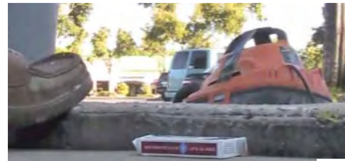
LOADING DOCK FLOOR Before (3" Drop)
