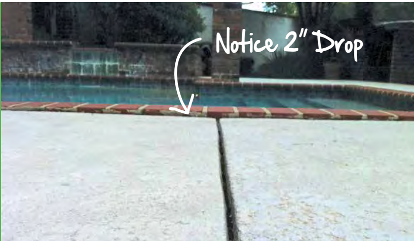
Before (Deck drop is unsightly and dangerous)
