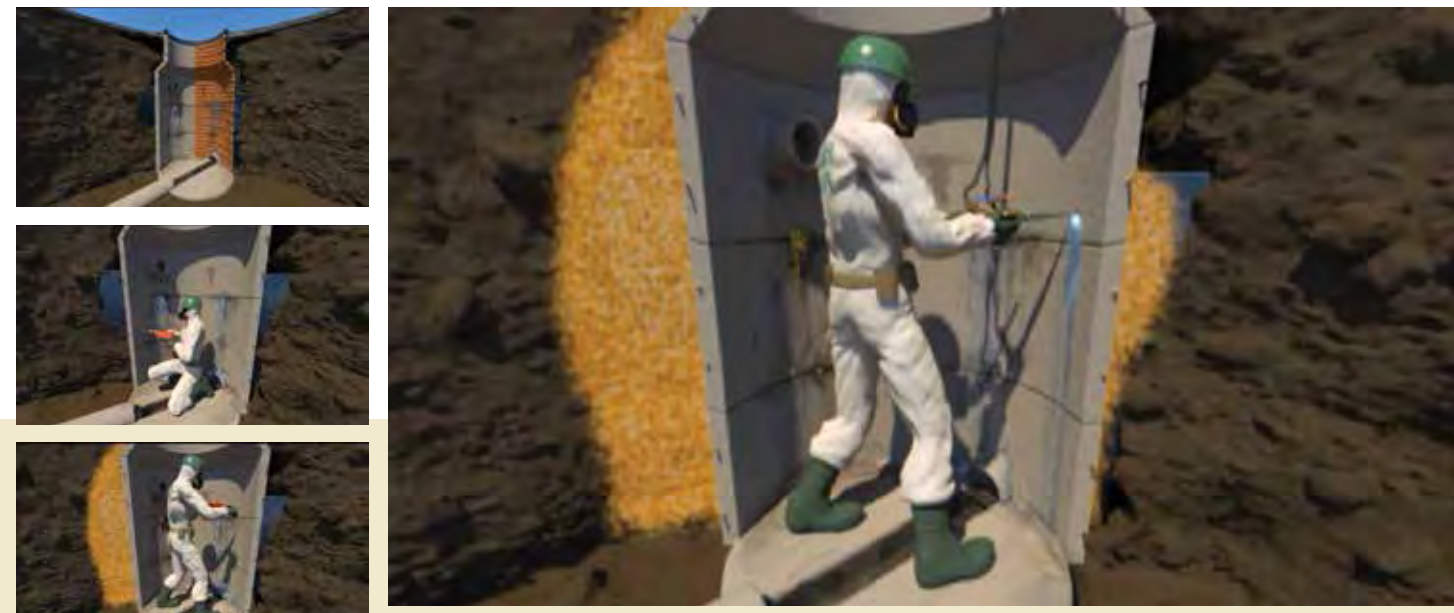
OUR PRECISION PROCESS OFFERS 50+ YEARS OF LEAK PROTECTION!
